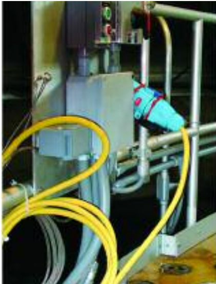
Connection to an Anaerobic Basin Mixer
